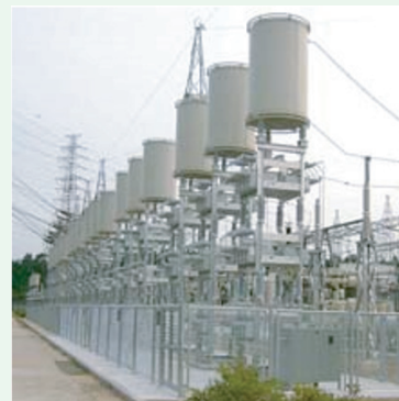
Figure TF26-2: A bank of large capacitors for three phase power. (Note the 3 lines going in and out of each capacitor.)
